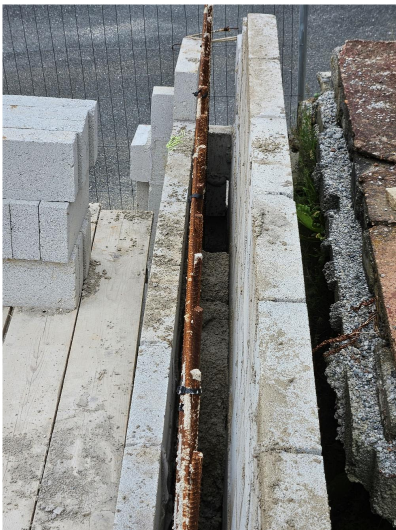
Photo 2 - Rear retaining wall, reinforcement in incorrect position
