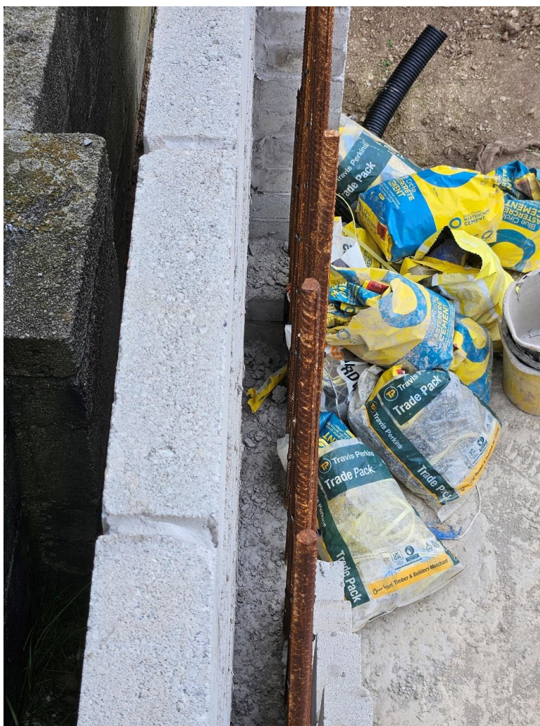
Photo 3 - Side retaining wall, starter bars not in correct position
